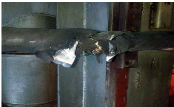
Figure 2. Breakdown of the medium voltage power cable at the bend point
