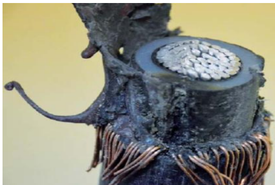
Figure 3. 10 kV cable after removing parts of the damaged coupling from it
