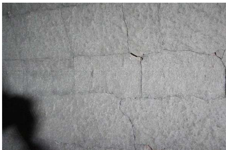
Fig. 4. The nature of lining destruction in the calcination zone
