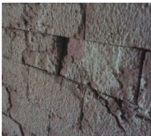
Fig. 2. Chipping on the inner surface of the lining of a sintering furnace.
